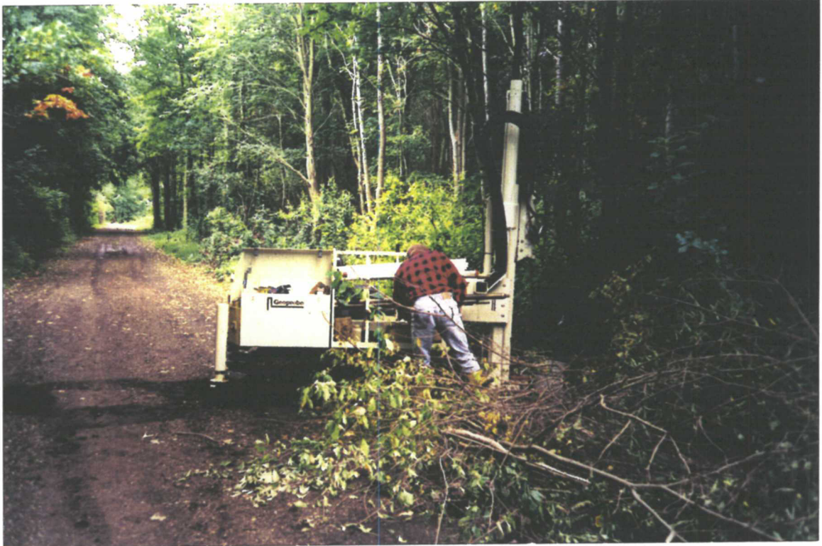
Photograph 7: Geogrobe sampling at downgradient location southeast of the former lagoon area (facing south).
